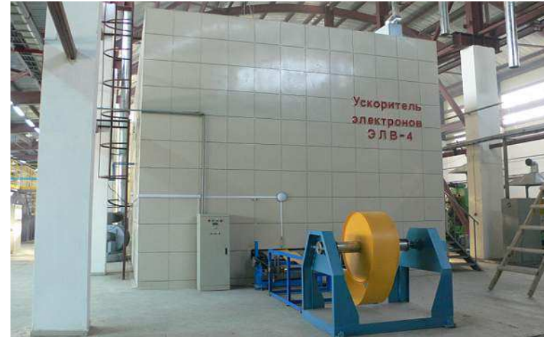
Electron accelerator bunker
